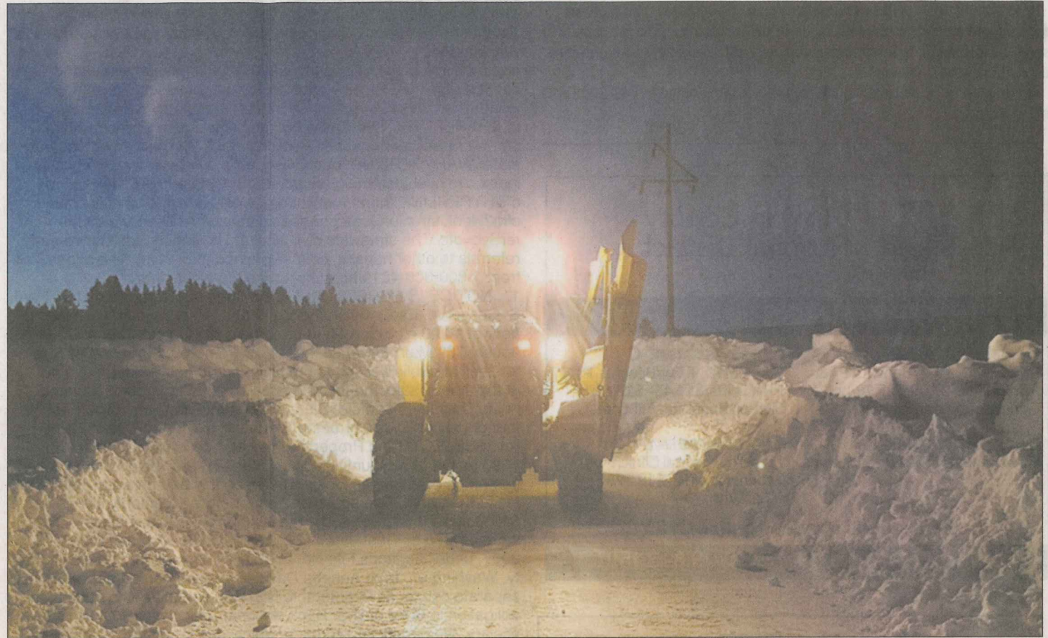
County equipment operator Willie Ruchert clearing Lewis Rd. south of the city.
