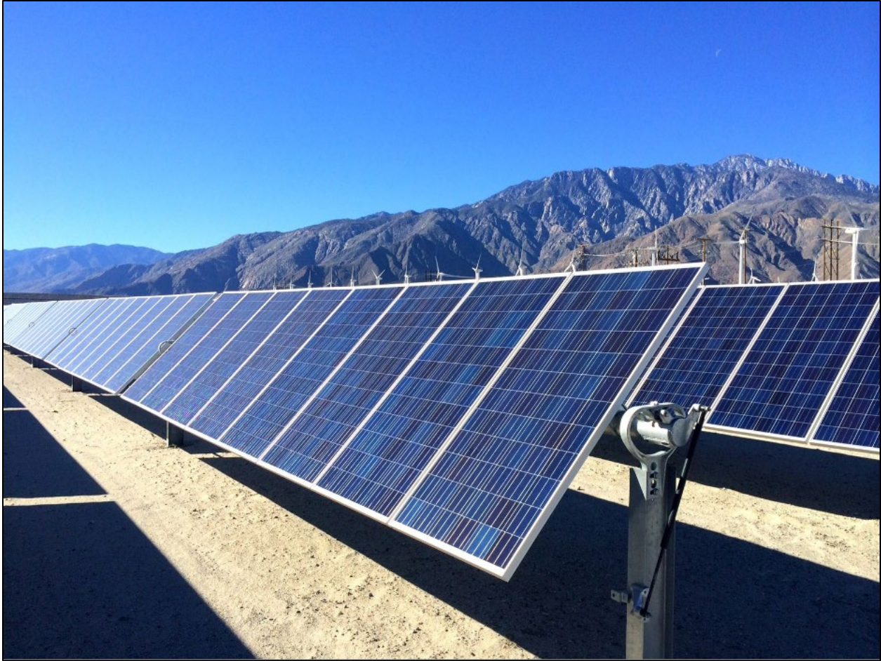
Figure 6. Example of solar arrays and panels.
